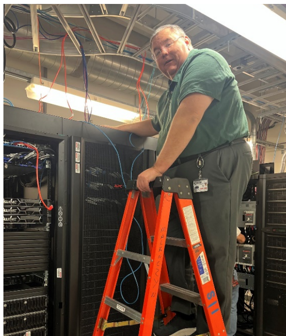
Wiring the networking for OwlCloud.
