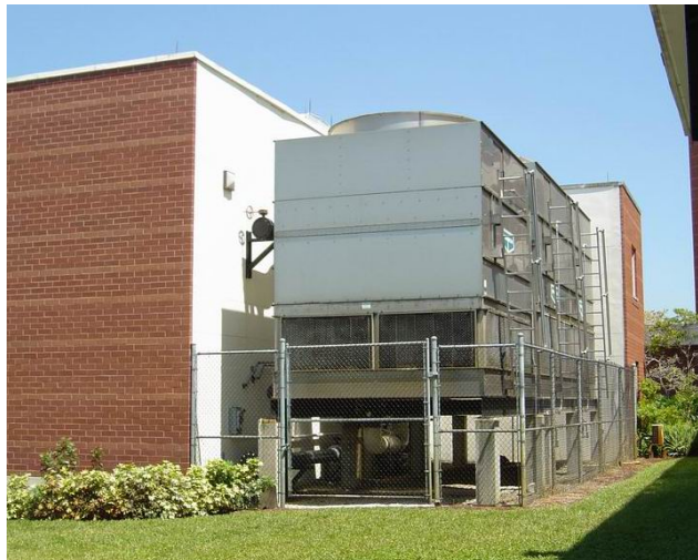
PHOTO 16.24 Fencing at the Chiller
